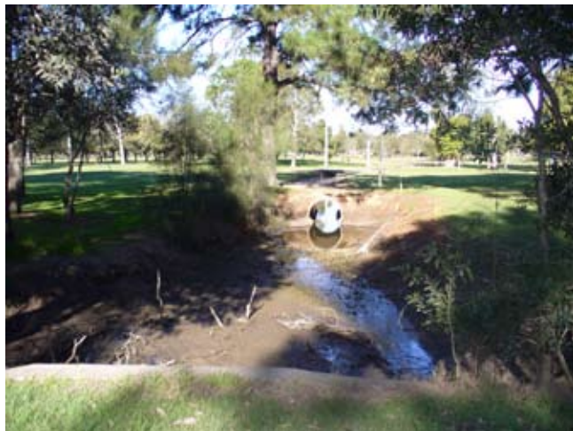
Plate 29. Stormwater pipes through golf course
