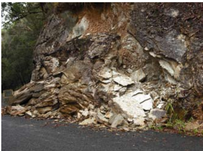
Plates 34 and 35. February 2009 Floods – South Arm Road
