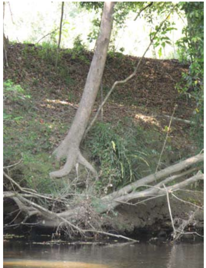
Plate 20. River bank erosion
