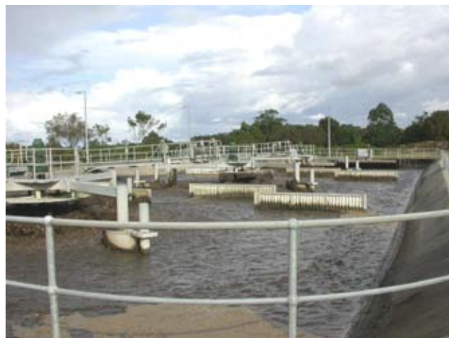
Plate 26. Urunga Waste Water Treatment Plant
